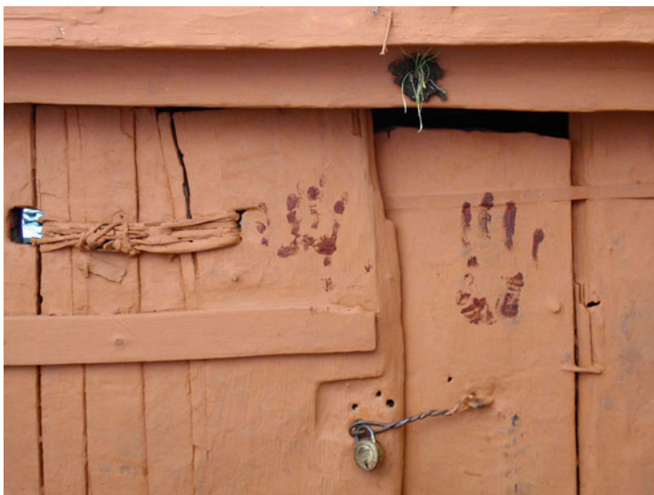
Fig. 3 Signs of protection. This door bears four signs of protection: ochre paint, two prints of a right hand on each side of the opening, a motif above the entrance, and a padlock. | © John Pavelka CC BY
